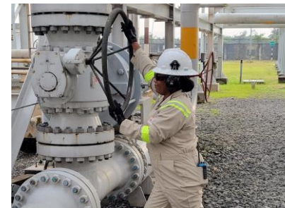
Rosiline Ini-Okor (Field Operator) operating a valve at the Uquo production facility in Nigeria.
