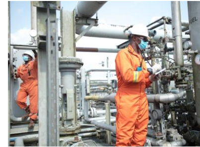
John-Mark Ogri (Maintenance Lead) and Osborn Essien (Senior Operator) at the Stubb Creek production facility in Nigeria.
